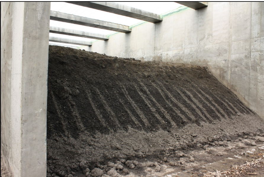
Inside an encapsulated bay. Note translucent roof panels to improve visibility for workers.
